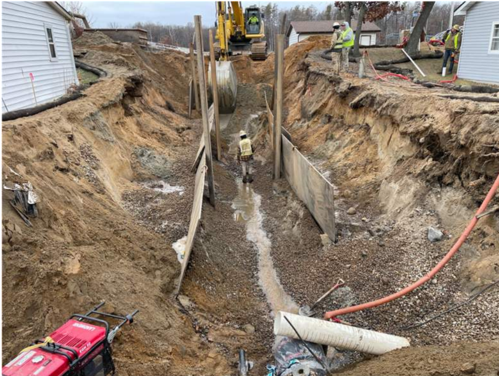
Photo #8: Preparing the bedding for the pipe to rest on from the inlet structure - Dec 8, 2023, 11:14 AM
