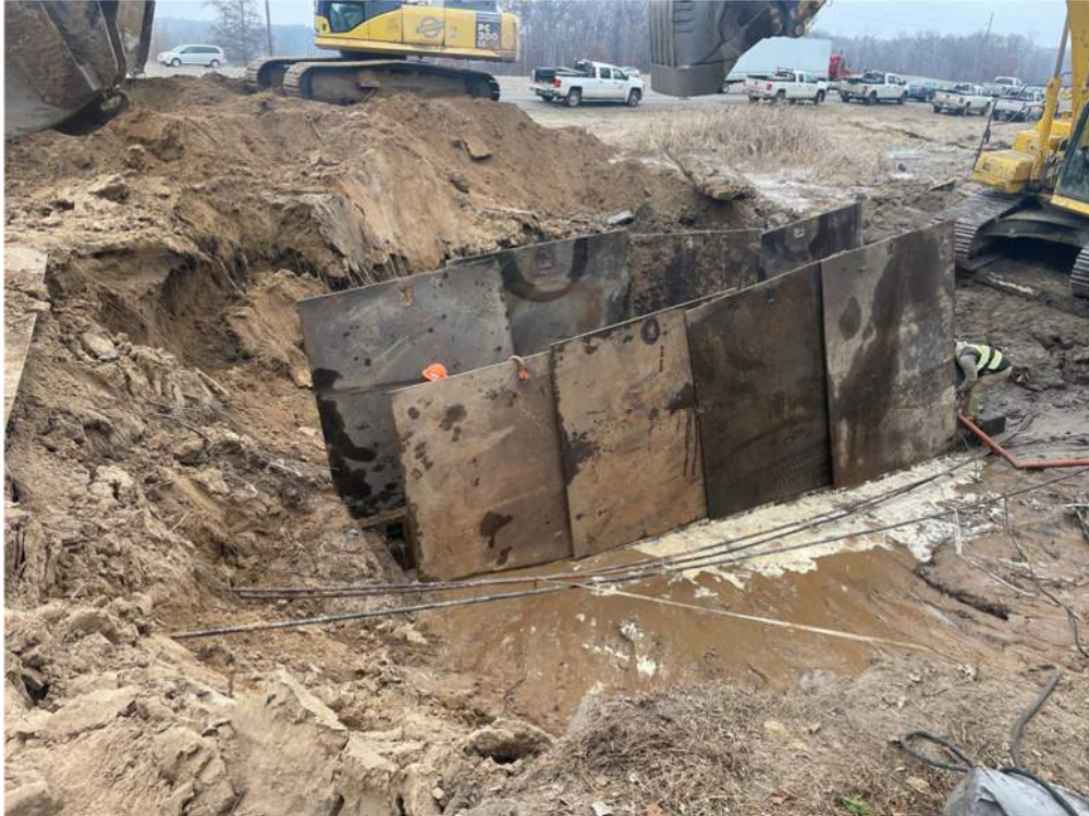
Photo #1: Additional sheeting added to the sides of the trench box to keep water out - Dec 4, 2023, 9:39 AM
