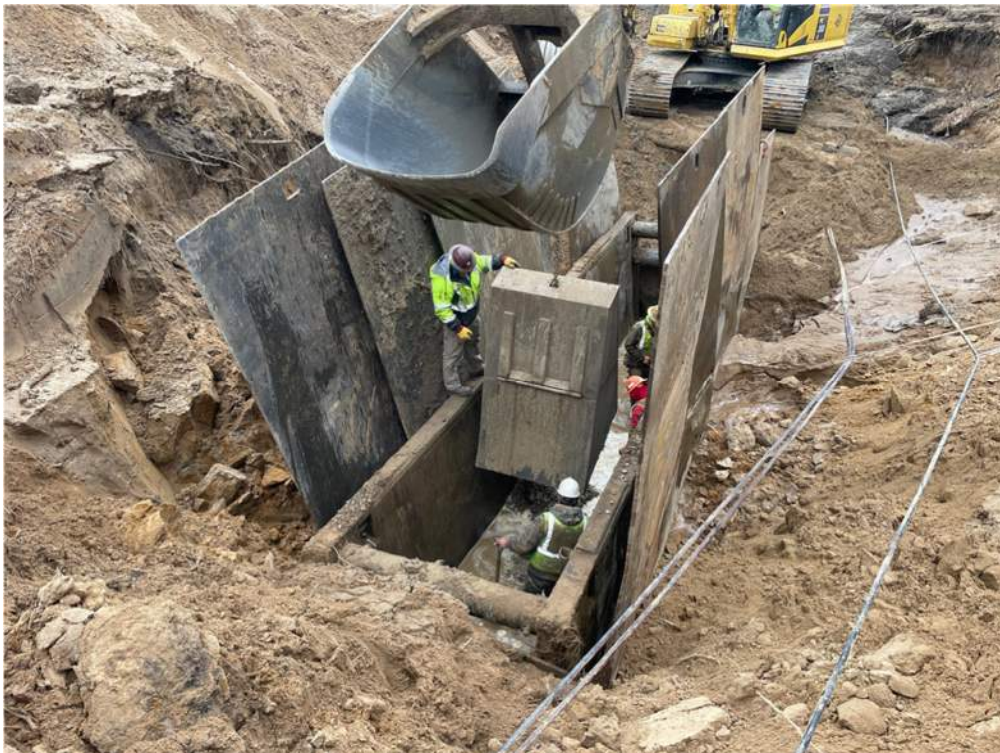
Photo #2: Moving metal doghouse to front of pipe to keep sediment and soil away and out of bell - Dec 4, 2023, 1:24 PM
