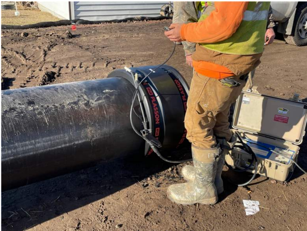
Photo #6: Fusing one side of the coupling to the 24" pipe - Dec 7, 2023, 11:12 AM
