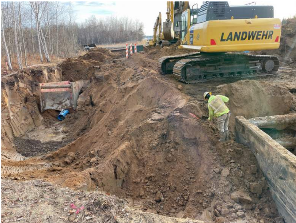
Photo #4: Excavating to connect force main at the southern part of the alignment alongside Highway 10 - Dec 6, 2023, 3:10 PM
