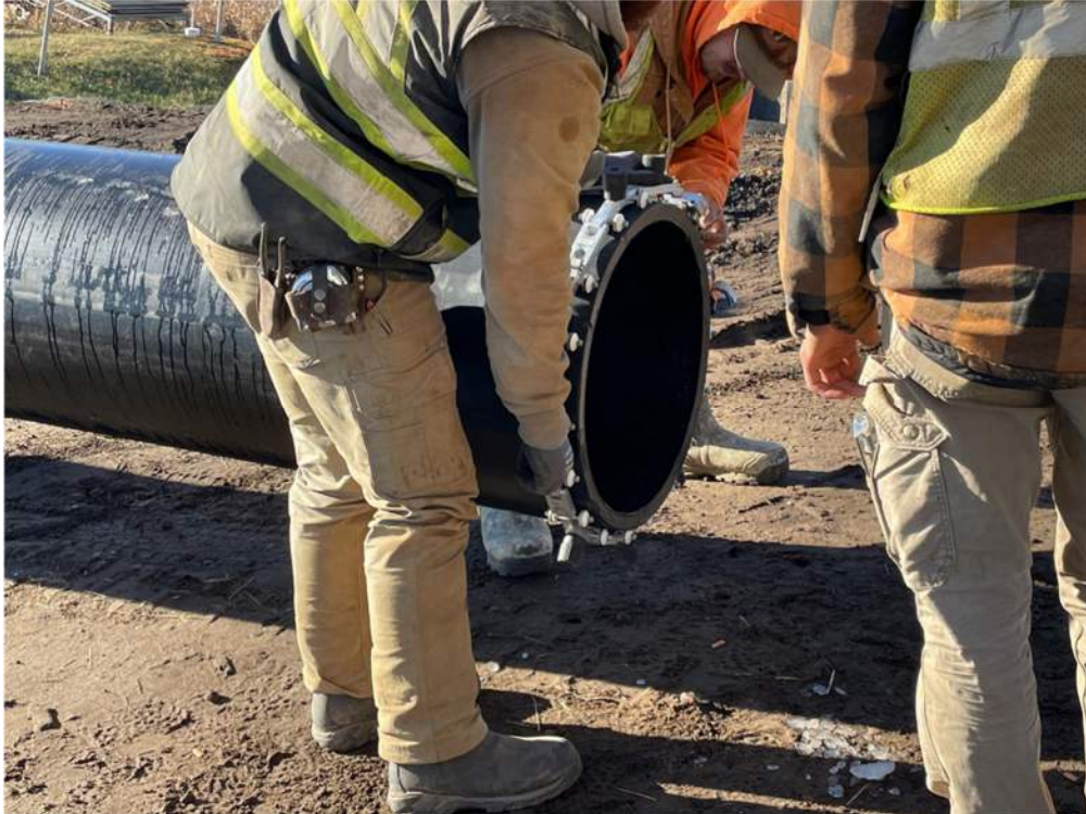
Photo #5: Rounding the end of the pipe to prepare it for fusing - Dec 7, 2023, 10:54 AM
